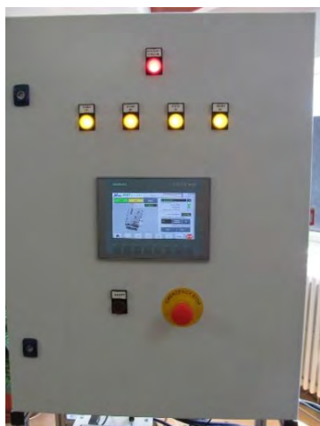
a- HMI display installed on the command-and-control panel
